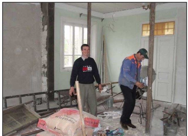
The interior walls have been torn down to provide a meeting room that will hold 100 Moldavians.
